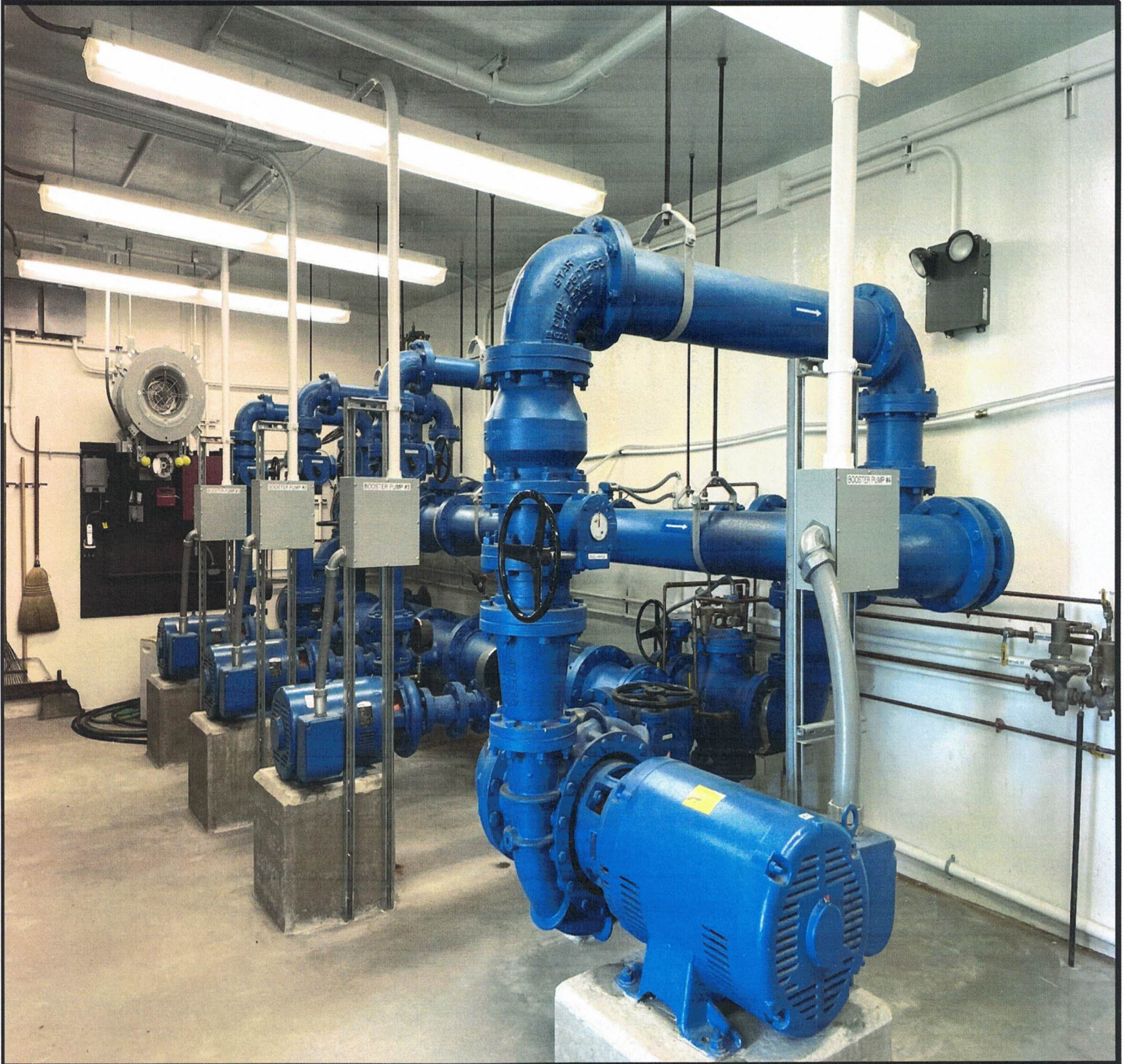
Interior of the Booster Station
